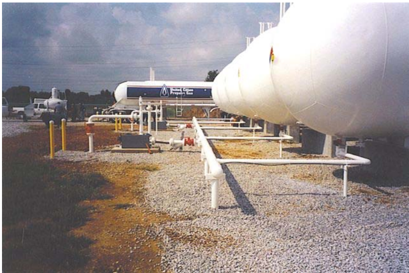
Local Fuel Storage
