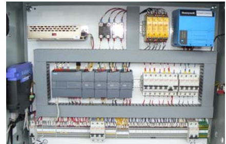
Standard Control Panel with Siemens S7-1200 PLC, Safety Controller, automatic circuit breakers, Ethernet Router, and Honeywell Flame Safeguard.
