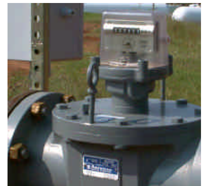
6 inch Flow Meter with direct Readout
