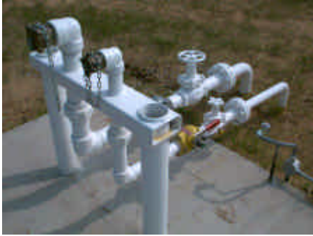
Typical Truck Unload Station with Nitrogen-operated ESV
