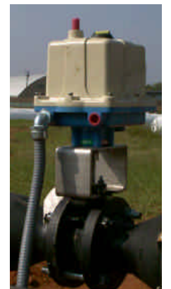
Flow Control Valve with Actuator for remote operation.
