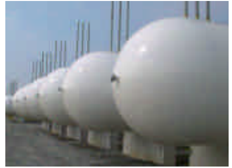
Typical Tank Farm with 30,000 gallon tanks
